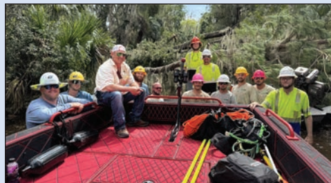
Crews had to navigate parts of Drayton and Hogg islands by boat during restoration.
