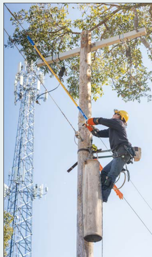
During a training exercise, Apprentice Lineworker Dalton Hollingsworth scales a pole for what's called a phase changeout, something he'll be tasked with performing at the rodeo.
