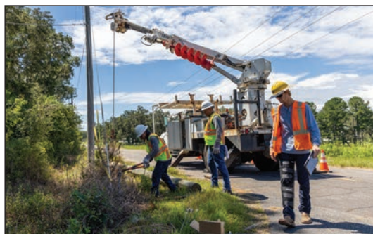
Clay Electric crews work to restore power following Hurricane Idalia in September 2023.
